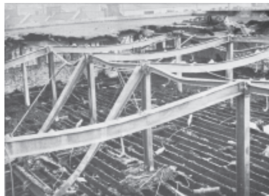
Fig. 04. Steel work affected by fire.
