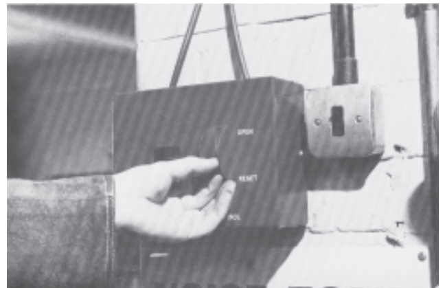
Fig. 11. Fireman's over-ride control for testing operation of fire vent installation, or for manual operation, when desired
